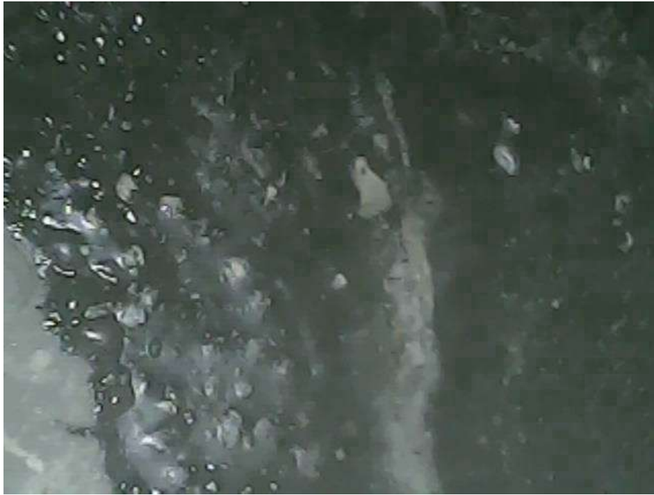
Photograph 35 – Bitumen leak to bearing shelf
