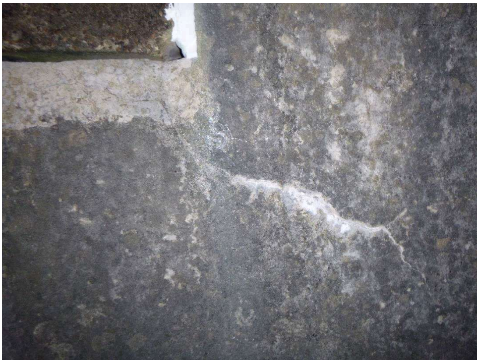
Photograph 14 - East joint south face crack
