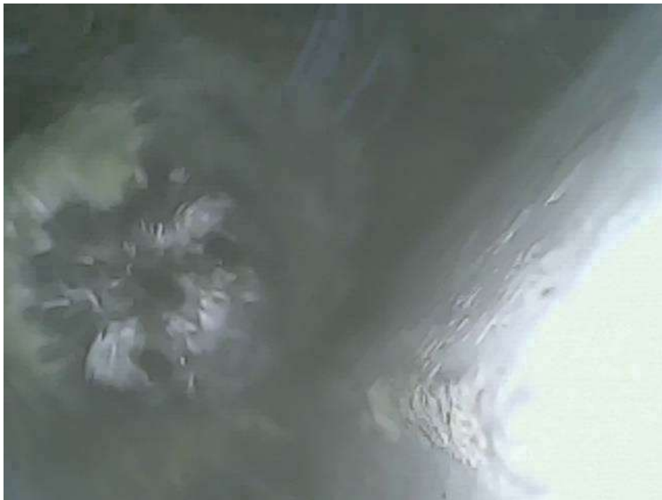
Photograph 20 – Active bird found nesting within half joint at south end.
