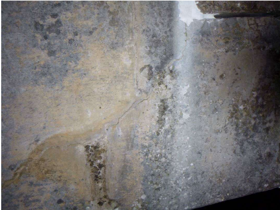
Photograph 15 - Crack on north face
