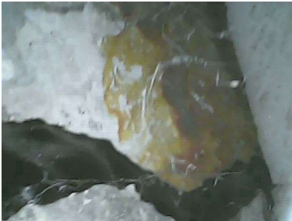
Photograph 18 - Leaking bitumen from surfacing expansion joint.
