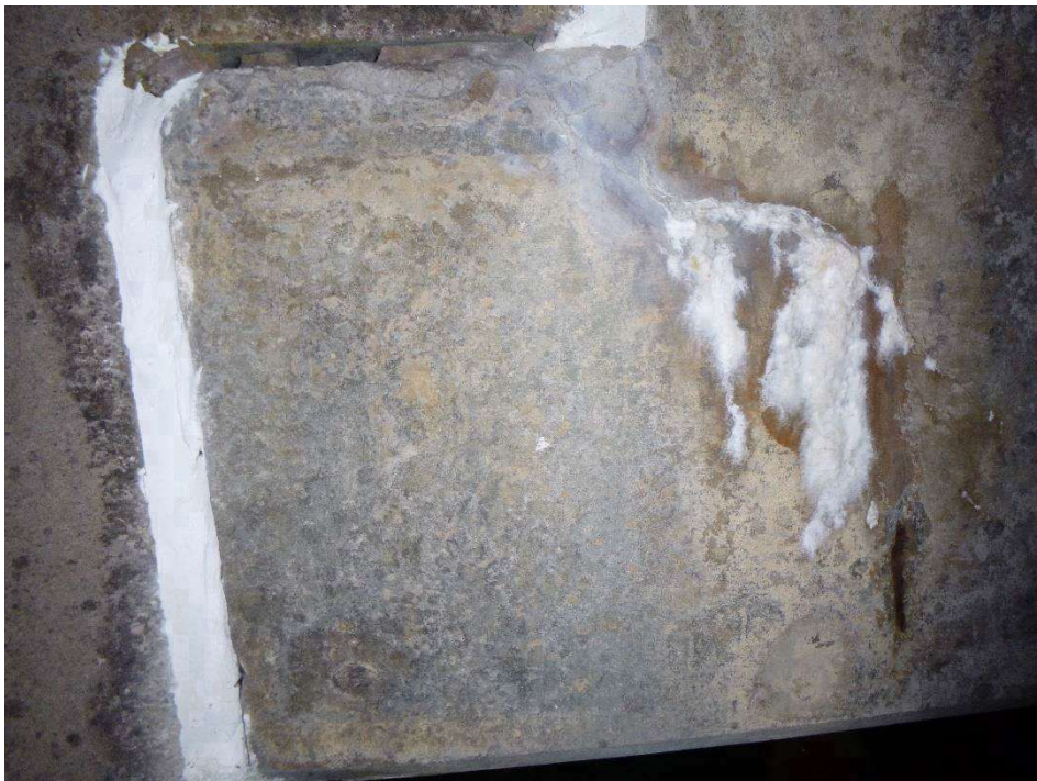
Photograph 32 - West joint north face crack
