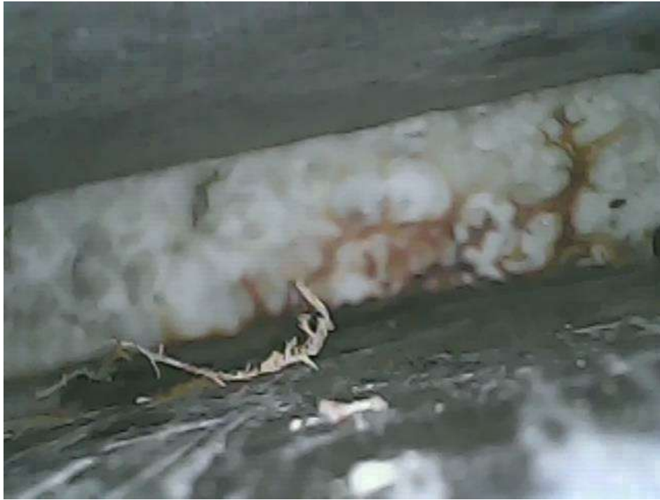
Photograph 11 - East half joint, polystyrene within joint
