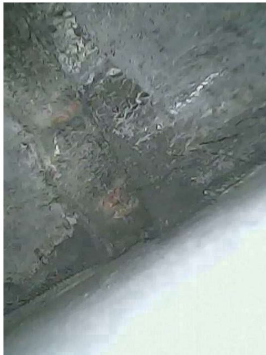
Photograph 36 – Perishing to bearing on north elevation.
