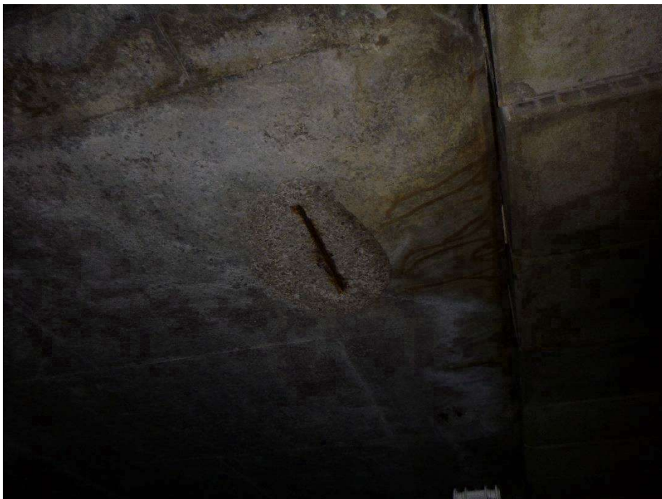
Photograph 34 - West half joint south side spall.
