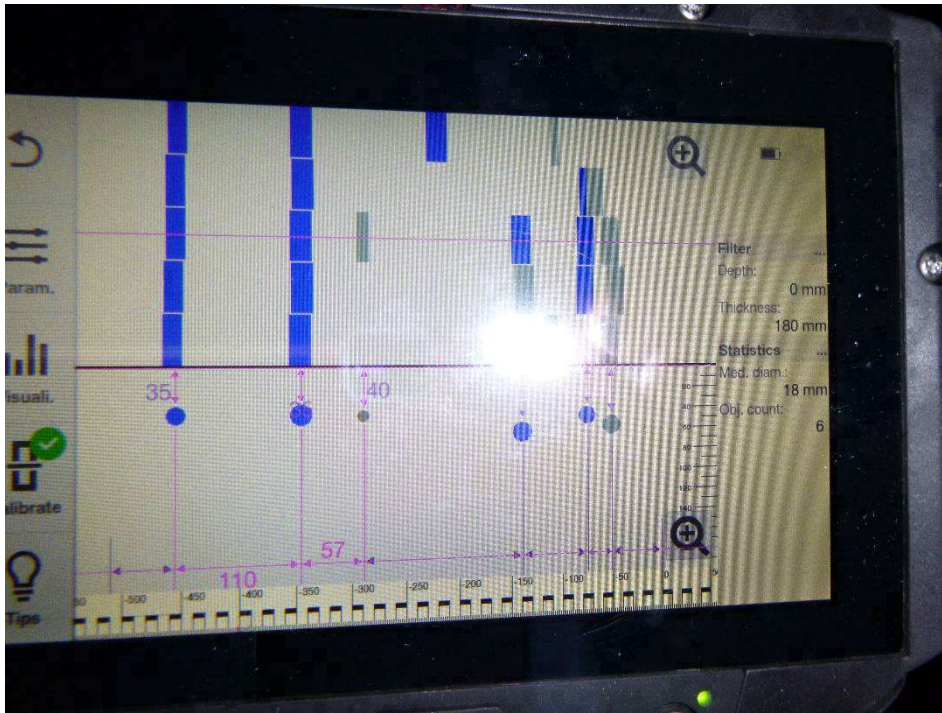
Photograph 41 - West half joint south face lower nib, scanned horizontally to show shear link reinforcement.
