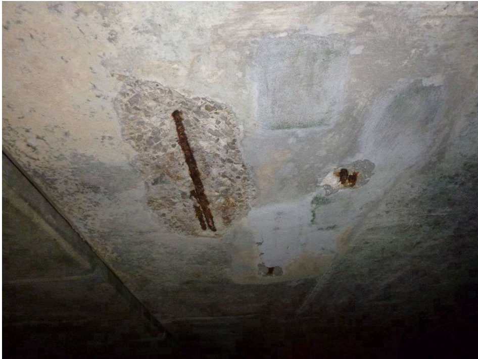
Photograph 33 - Spalling to soffit of cantilever.
