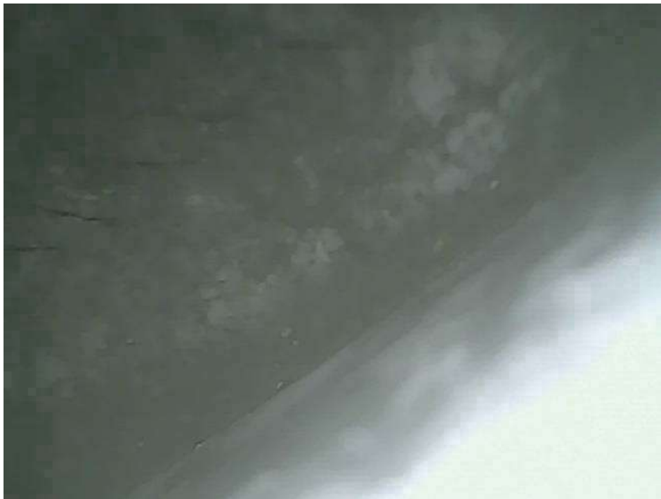
Photograph 22 - Cracking to bearings within half joint.
