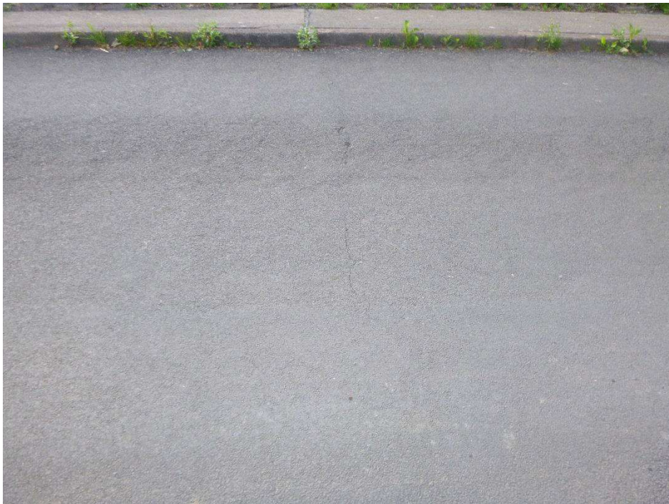
Photograph 8 - Cracking to carriageway local to east half joint.
