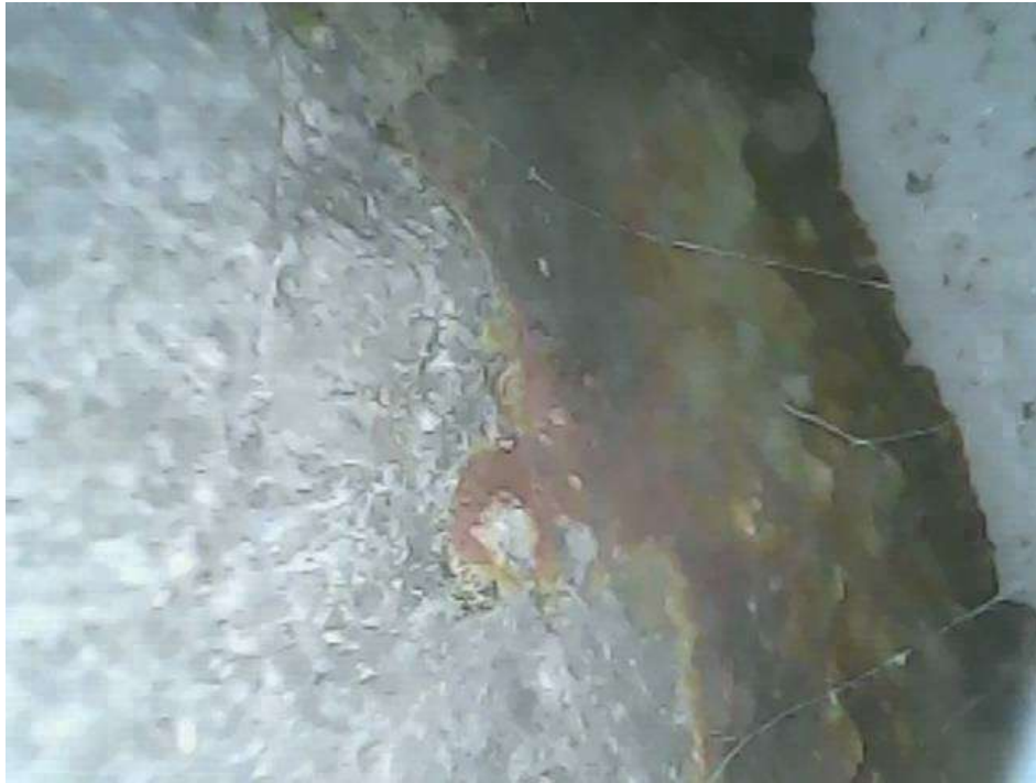
Photograph 17 - Localised corrosion staining to bearing shelf corner.
