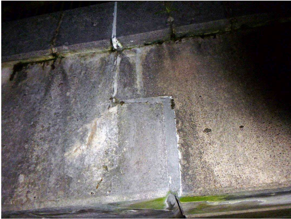
Photograph 29 - West joint south side elevation. Note, hairline crack xxmm wide.
