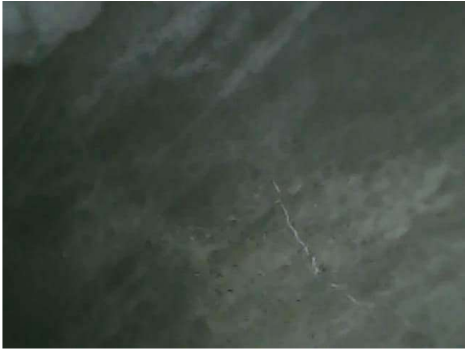
Photograph 21 - Crack to lower nib (north elevation)
