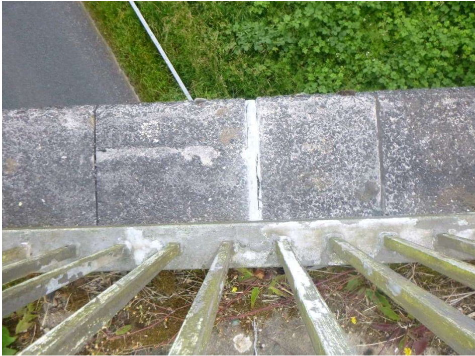
Photograph 31 - Cracking to sealant at west half joint
