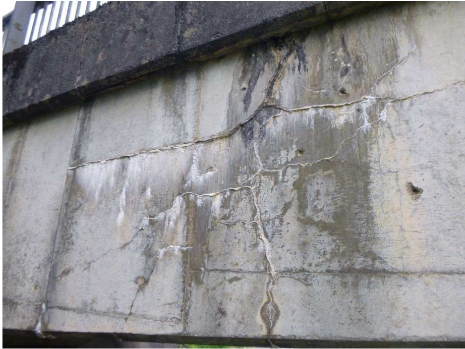
Photograph 25 - Cracking to deck cantilever behind half joint (not associated with half joint)
