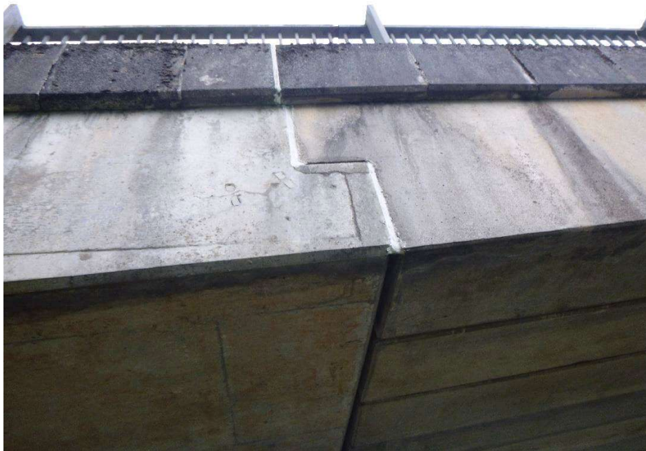
Photograph 14 – North-east half joint
