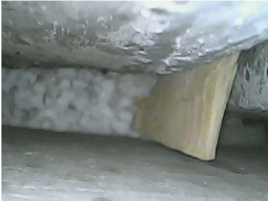
Photograph 13 - Timber and polystyrene between edge box beam and internal beam around diaphragm cap.
