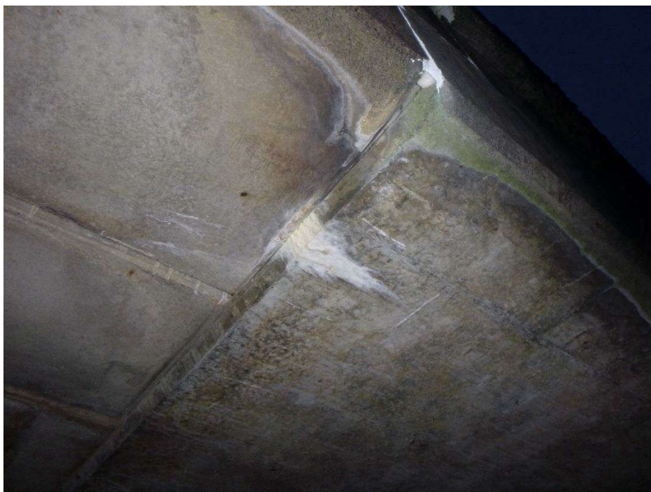
Photograph 20 - Leachate staining to cantilever soffit.
