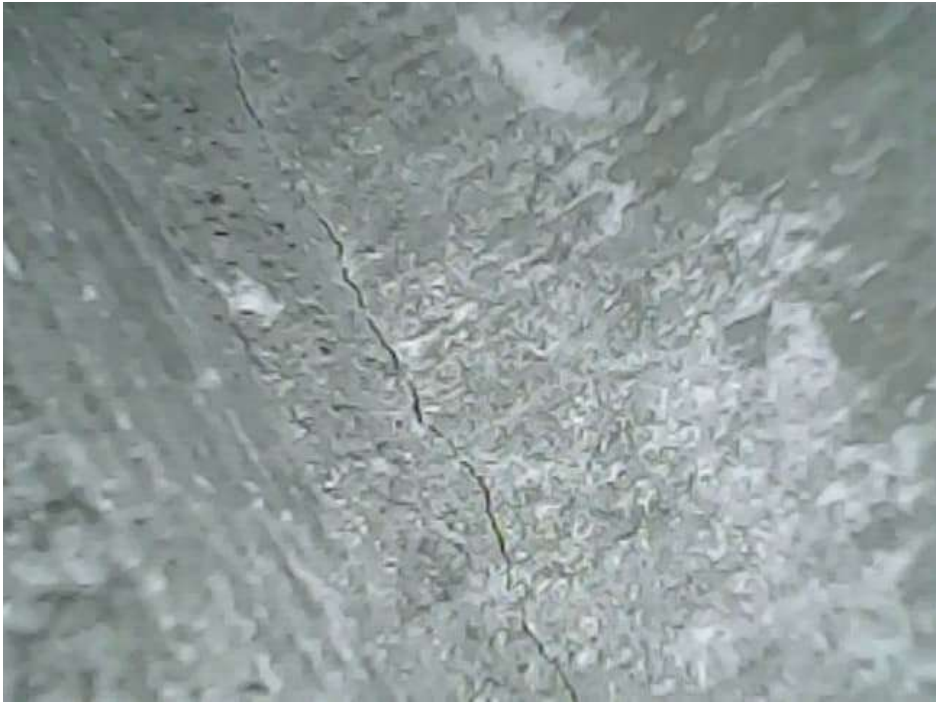
Photograph 23 - Crack to lower nib (2 nd beam from south)
