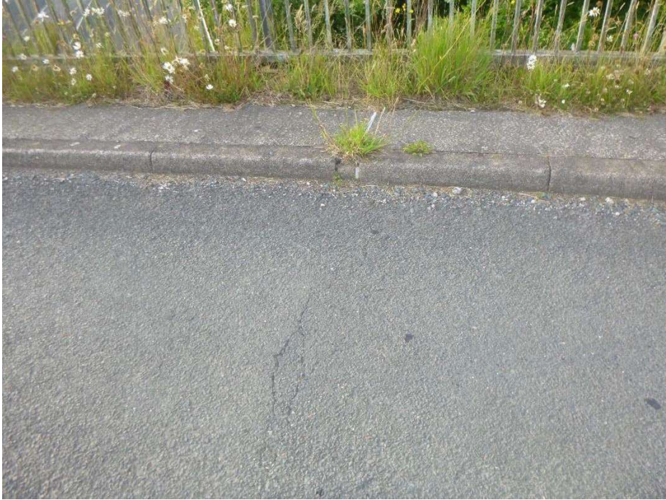
Photograph 9 - Cracking to north side of carriageway at east half joint
