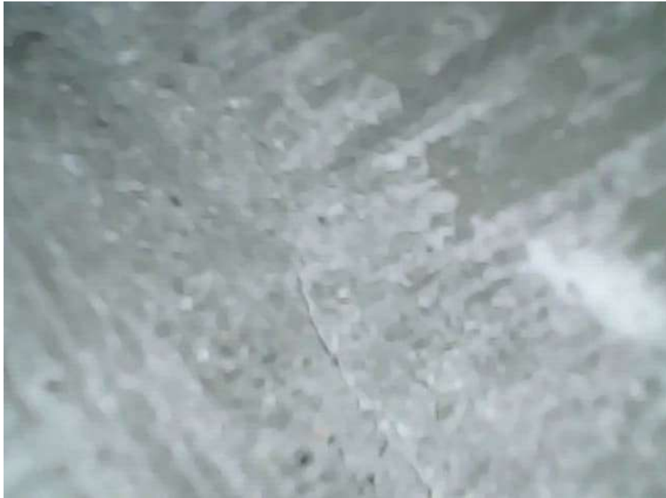
Photograph 17 - Crack to upper nib (2 nd beam from south)
