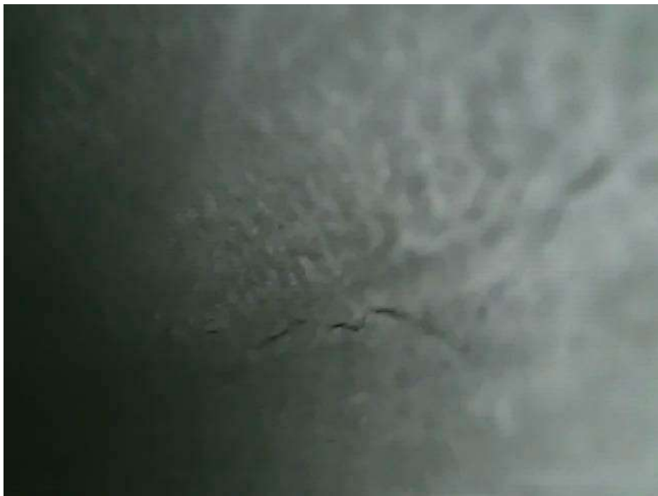
Photograph 22 - Second crack to lower nib
