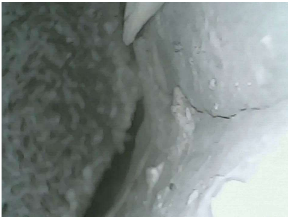
Photograph 16 - Narrow crack to upper nib of T-beam (3 rd from north)
