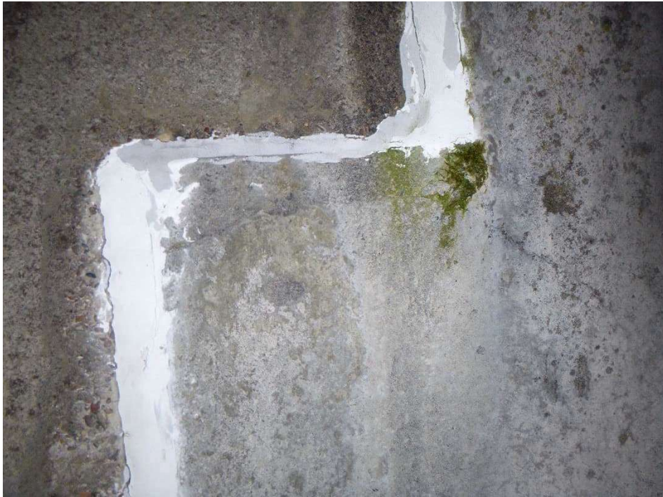
Photograph 37 - Algal staining and previous repair to north-west half joint. Note, the joint is fully sealed.
