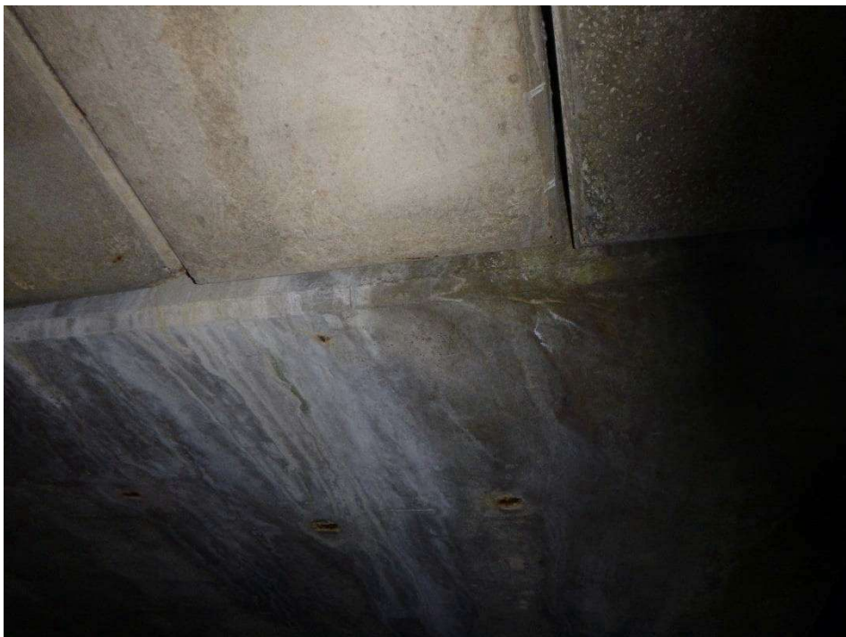
Photograph 38 - Leachate staining to deck soffit.
