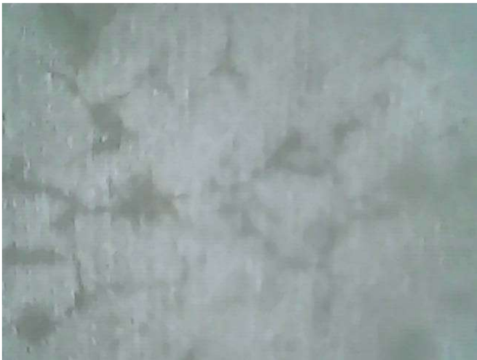
Photograph 36 - Shrinkage cracking to northern T-beam upper nib.
