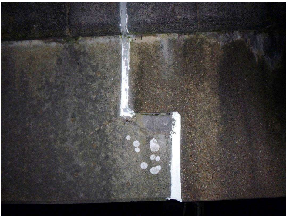
Photograph 34 – South-west half joint. Note, previous repair and minor spalls.
