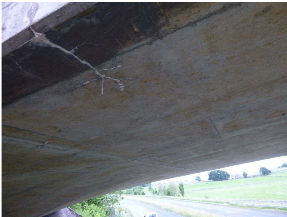
Photograph 26 - Cracking to deck cantilever soffit behind half joint (not associated with half joint)
