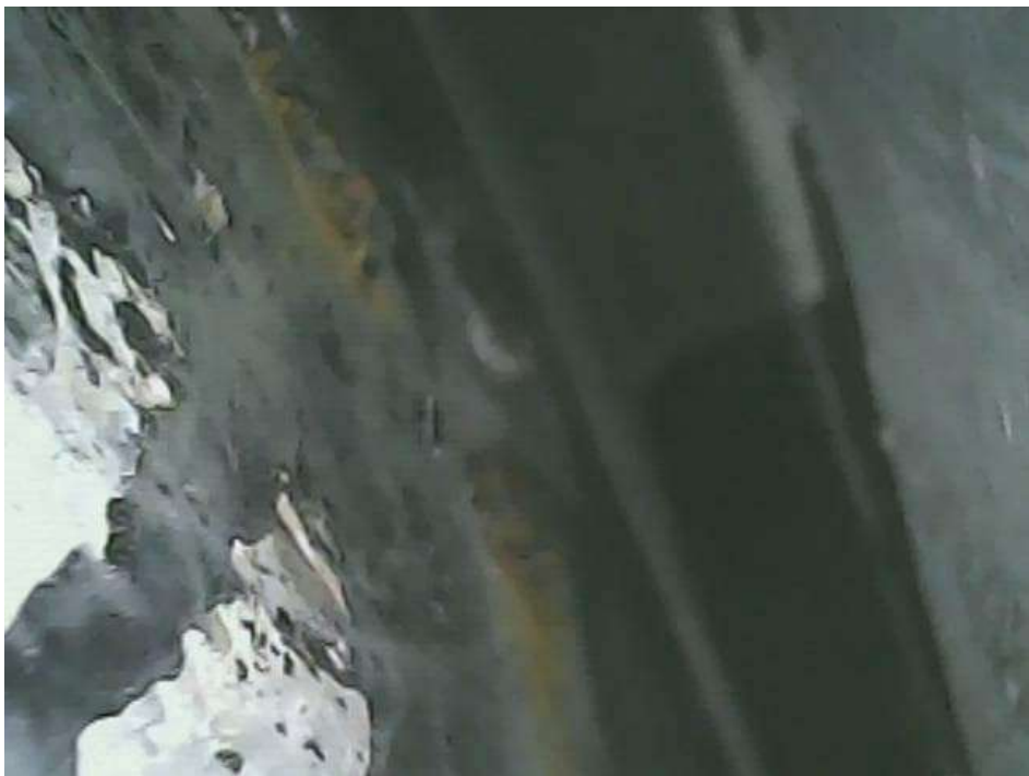
Photograph 40 - Bitumen leak and rust staining between south beams
