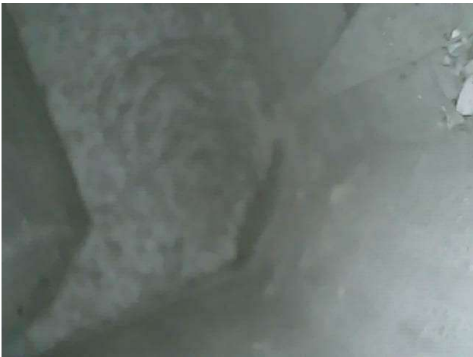
Photograph 12 - Polystyrene in joint
