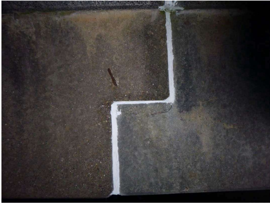
Photograph 15 – South-east half joint. Note, previous repair and exposed reinforcement.
