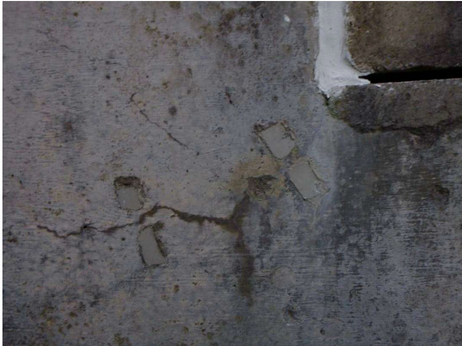
Photograph 19 - Close up on cracking to north-east half joint
