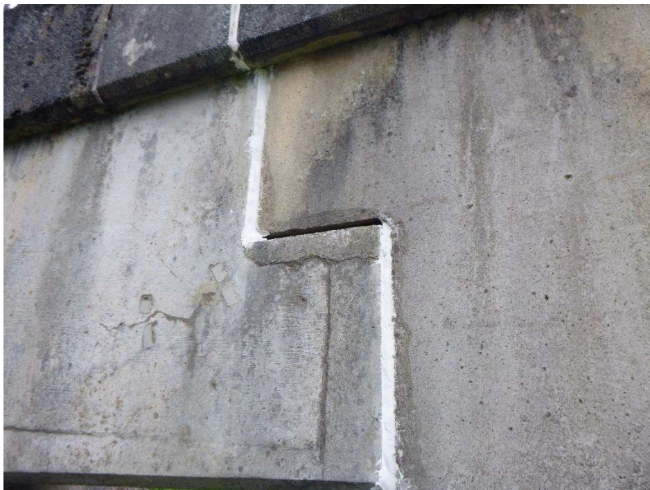
Photograph 18 - Cracking and previous repairs to north-east half joint
