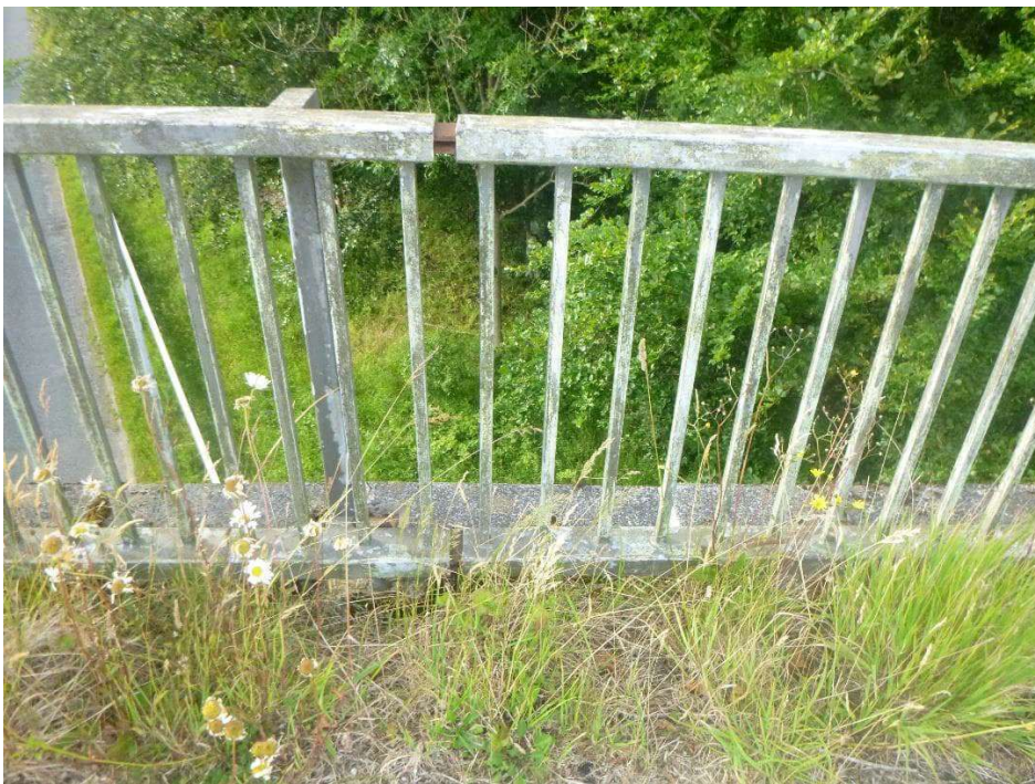
Photograph 10 – South-east parapet expansion
