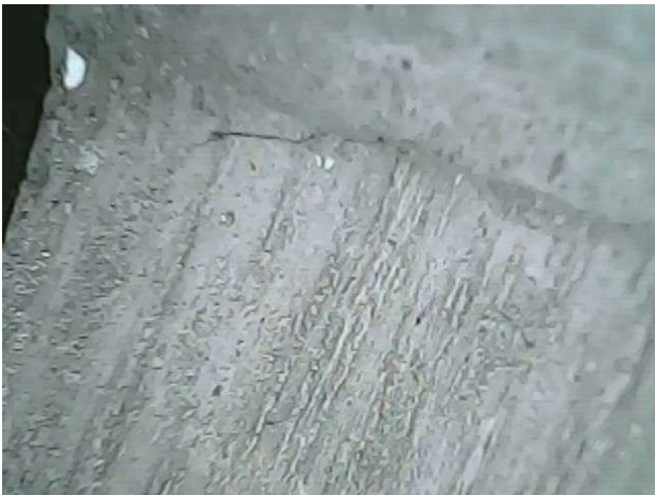
Photograph 24 - Crack to lower nib of south box beam.
