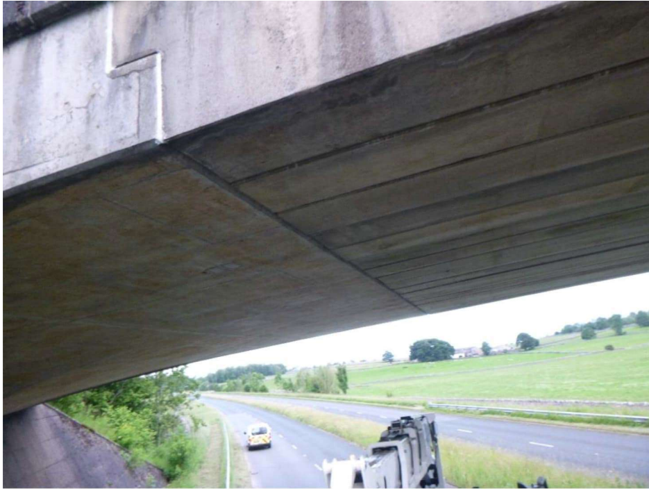
Photograph 5 – View along east half joint showing poor alignment of deck beams.
