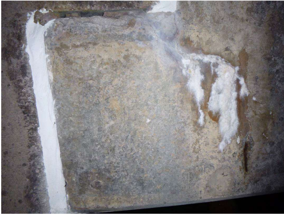
Photograph 3 - West joint north face crack
