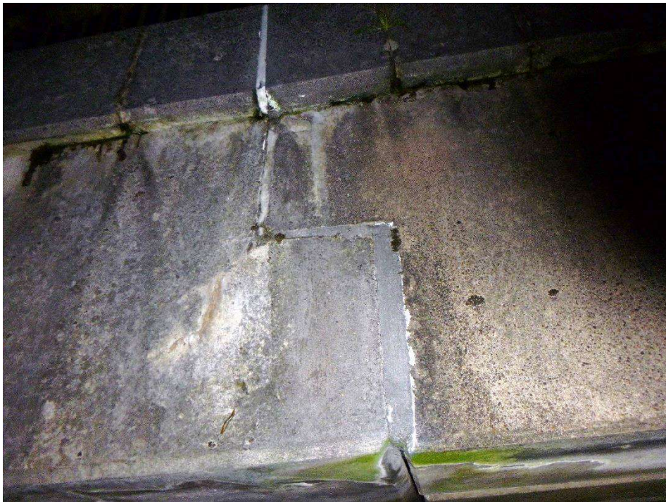
Photograph 4 - West joint south side elevation. Note, hairline crack.
