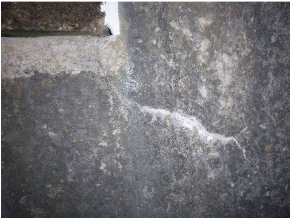
Photograph 2 - East joint south face crack
