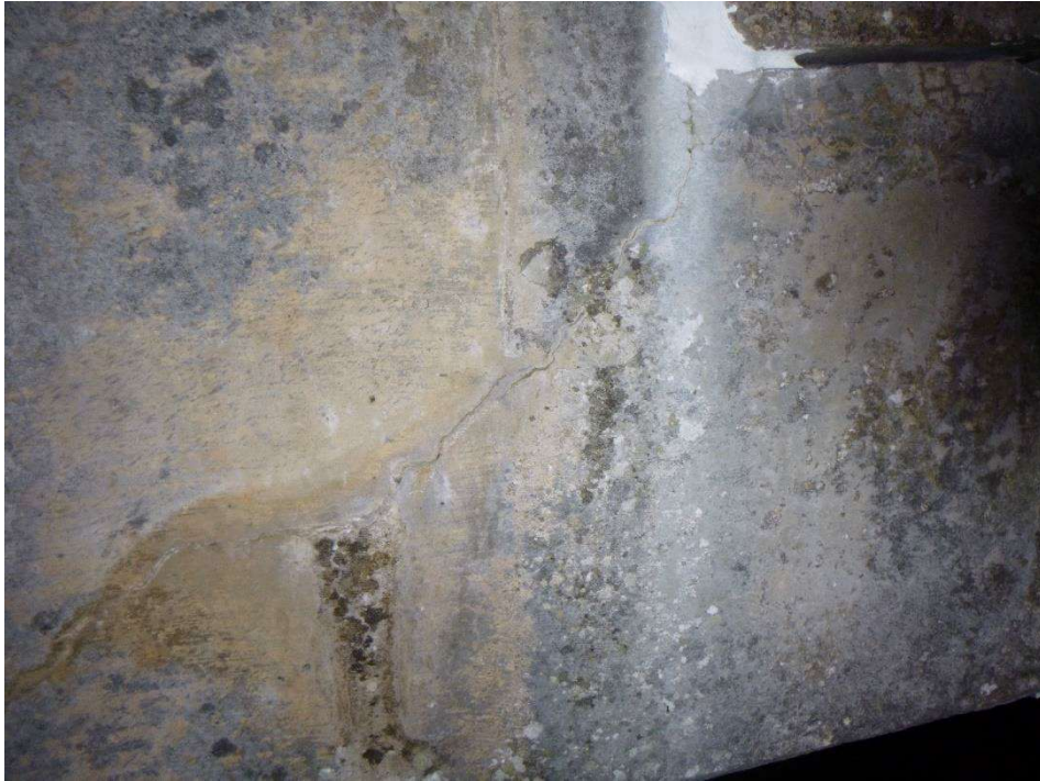
Photograph 1 - Crack on north face
