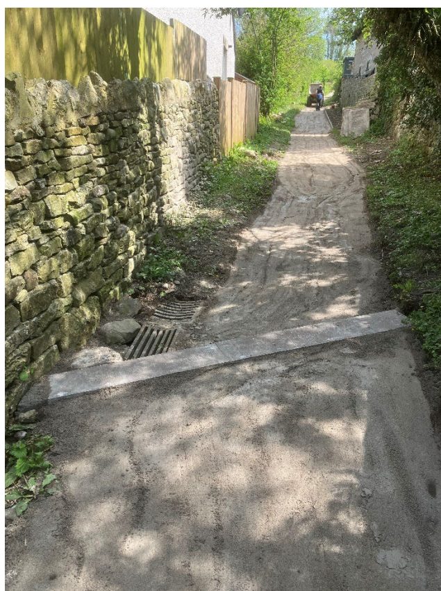
Figure 2: Public right of way improvement, north of Boon Town housing development to A6070, Burton-in-Kendal.
