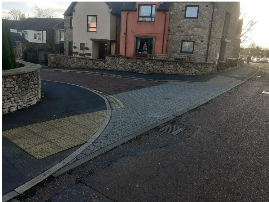
Figure 4: Resurfacing of footways and carriageway in the vicinity of Waterside Estate, Dowker's Lane, Kents Place, Bishop Court in Kendal.
